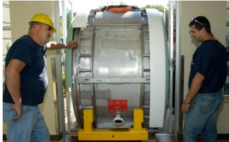
MAGNETOM ESSENZA delivered through the front doors at Battlefield Imaging.
