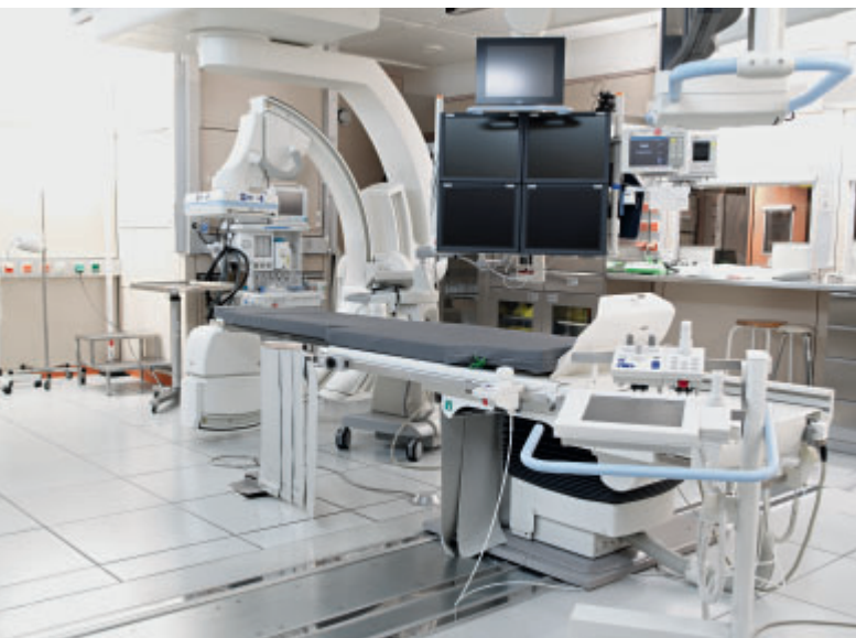
Installation of Angio-MR MIYABI at the AKH. The angio table travels on rails to the MRI.
