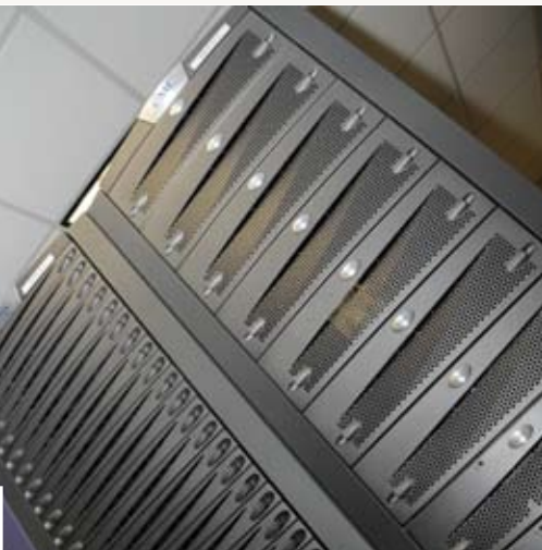
One of two EMC Centera content-addressed storage systems installed in the Children's data center.
